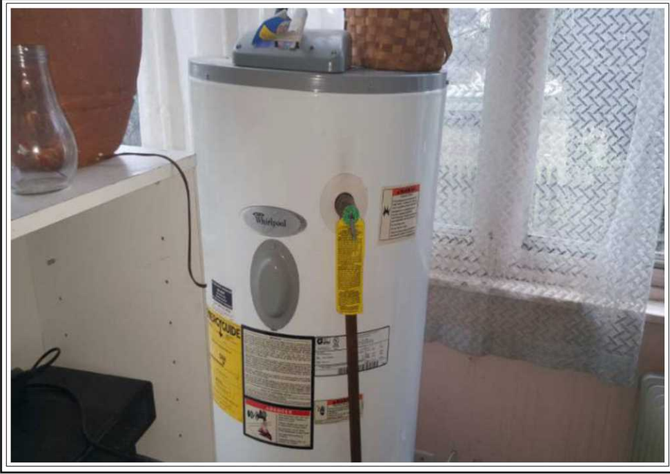
Hot Water Heater
